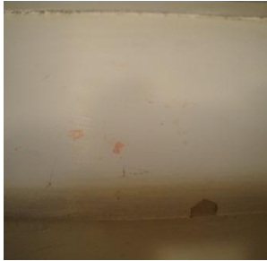
Further Marks on Window Sill and Chip
